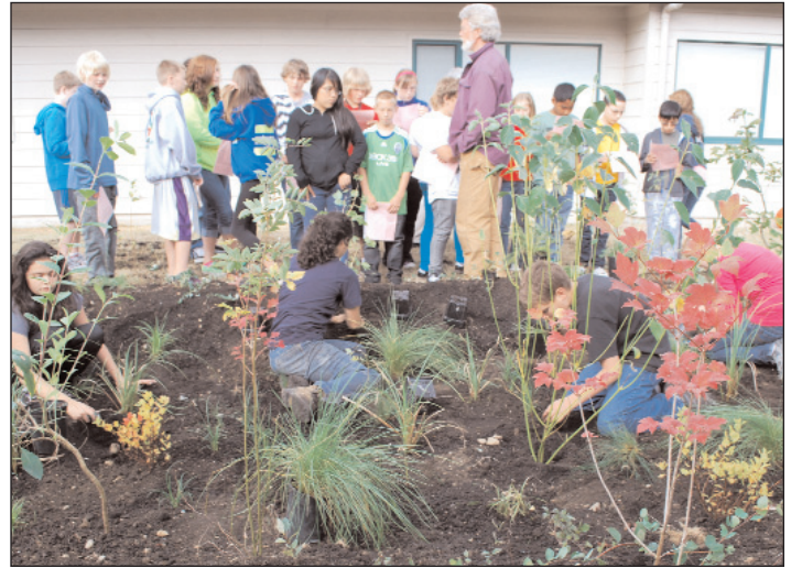
Cedar River Middle School students, under the direction of Peter Donaldson, of Friends of the Cedar River Watershed, construct the school's first rain garden, which creates a natural filter for polluted rainwater from the school's roof.
